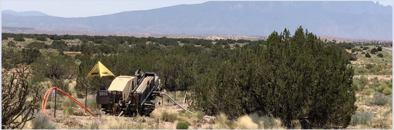
Kelly Cable of NM Directional drilling equipment utilizes trenchless technology on the Jemez-Zia project to install the conduit for the fiber optic cable across rugged terrain, such as arroyos, or under roads.
