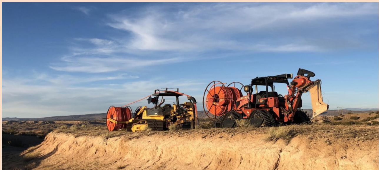
Ploughs are able to 'sew' the conduit into the ground by cutting a 6" opening to lay the conduit at depth without the labor costs and invasiveness of a backhoe to complete the same job.
