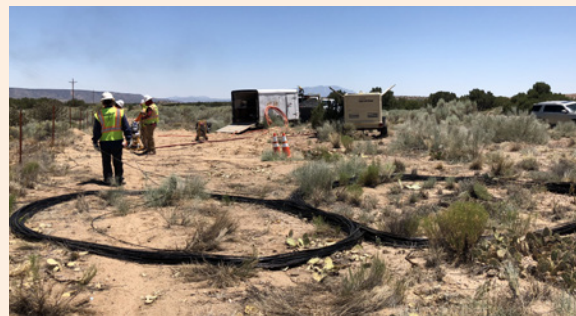
Fiber crews coil the fiber optic cable in large figure eights in preparation to blow the fiber between pull boxes located approximately 2000' feet apart. The process is repeated every 1-2 pull boxes for the 30-mile route.
